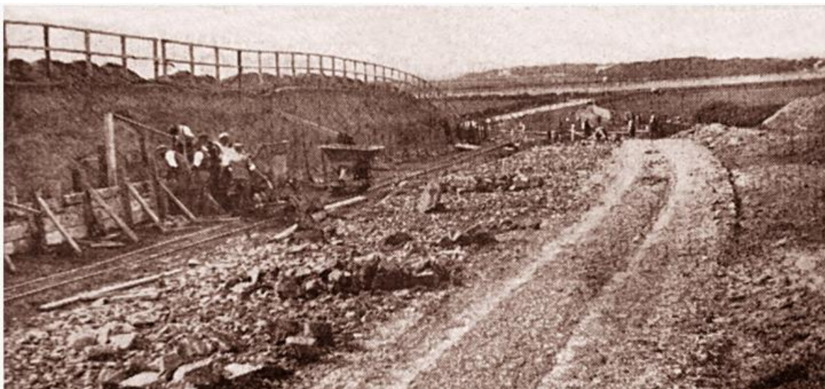
August 1929 Caption "Road Improvements. View on the new Thornton to Fleetwood Road. The hill on the left has been cut through." (Unattributed photo, discovered by Ted Lightbown)
