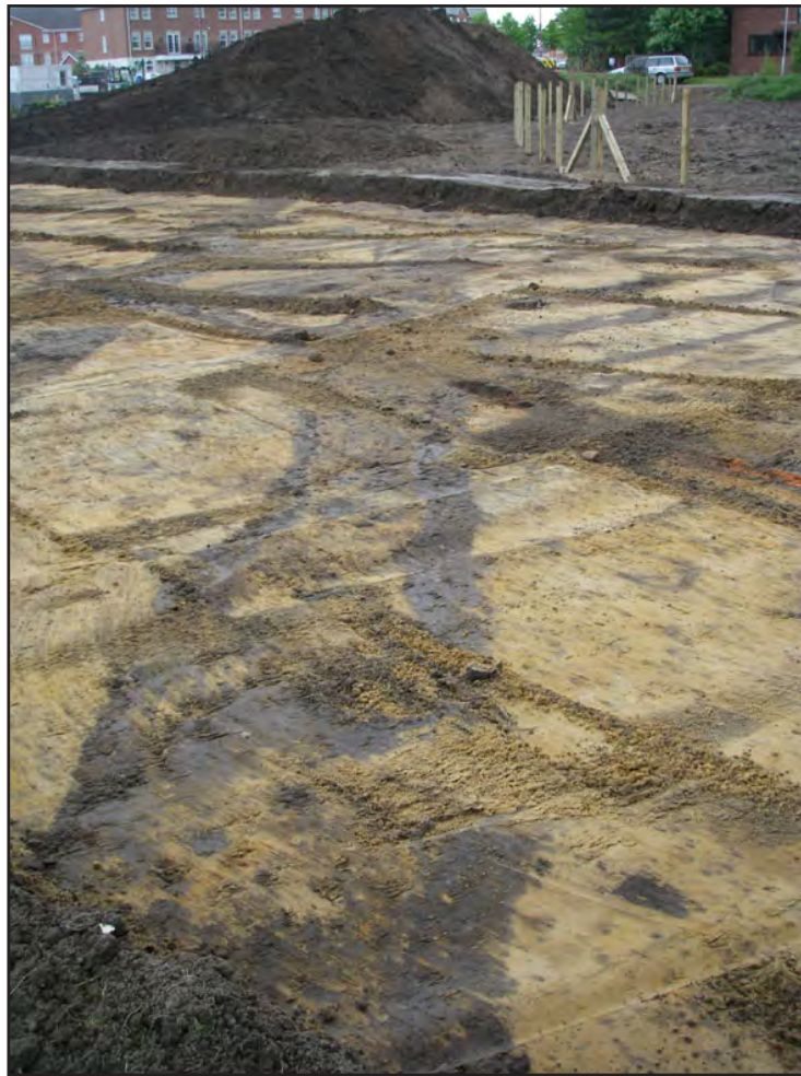
Plate 3. Modern pipe trenches within the western part of the stripped area, looking southeast
