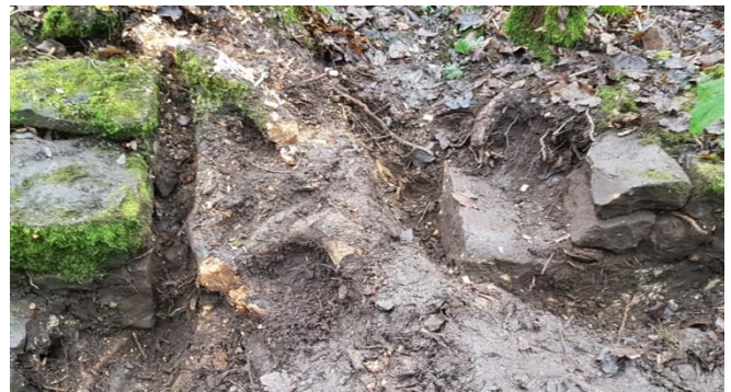
Dave and Andy revealed what appears to be a doorway in the south wall. Tree roots are a major obstacle.
